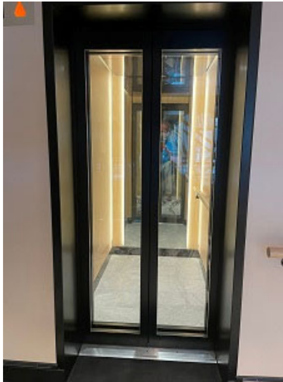
ONE OF TWO ELEVATORS
